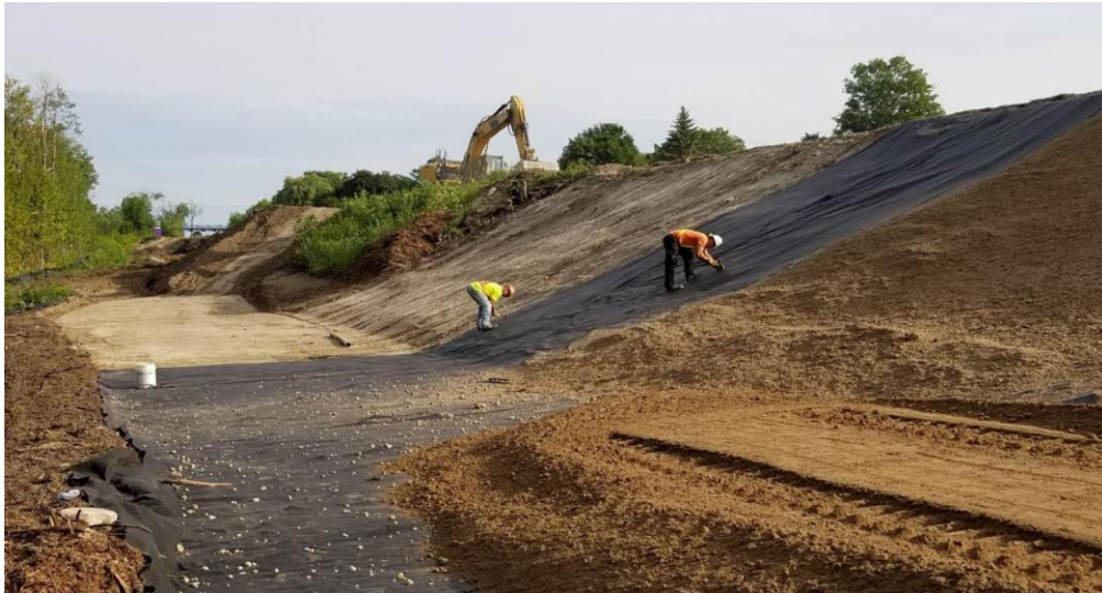
Work continues along the Earth Dams south of Parkhill road in Peterborough
